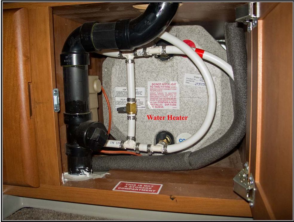
Picture W-16: Water Heater Compartment
