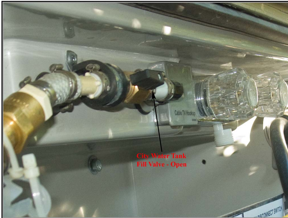
Picture W-7: Open position of the city water tank fill valve.
