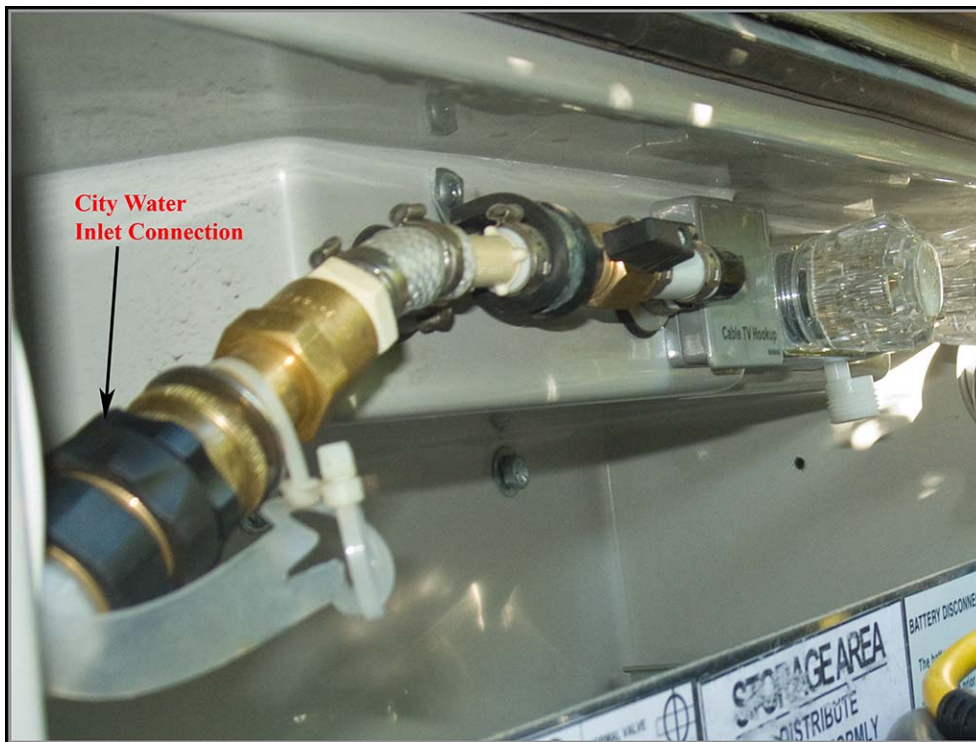
Picture W-6: Location of the city water inlet connection.
