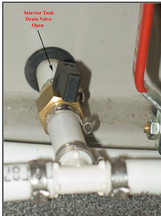
Picture G-12: Interior tank drain valve in open position.
