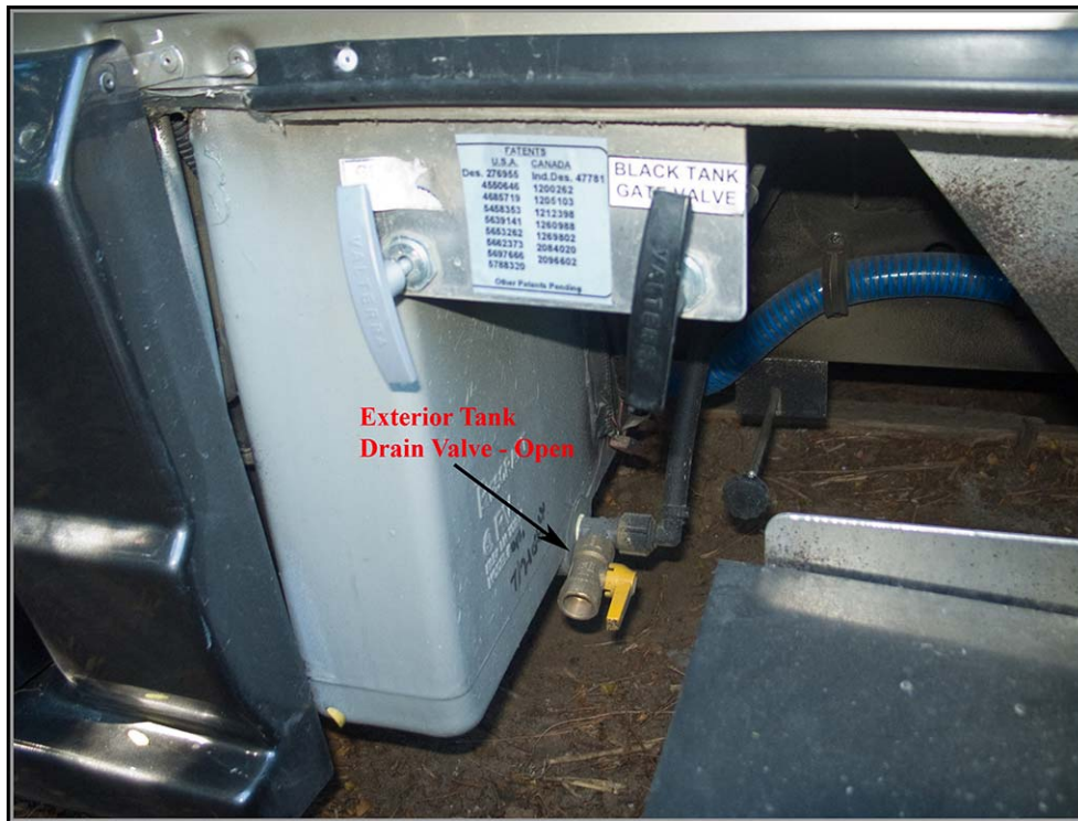
Picture W-14: Exterior fresh water tank low point drain valve.
