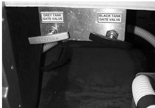
Picture G-P14: Access to sewer discharge assembly, black and grey gate valve handles.
