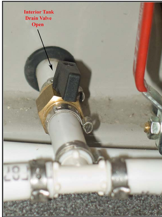
Picture W-10a: Interior Tank Valve in Open Position
