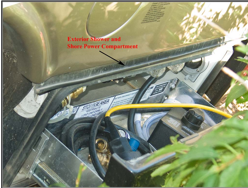
Picture W-9: Outside shower and shore power connection.
